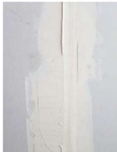
5 Filler is applied generously to allow for an even distribution along the length of the joint.
