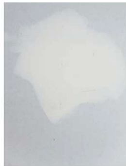
8 Sanding smooths and evens off the filler and reduces it to the level of the plasterboard. When painted, variation in level and texture will be invisible.
