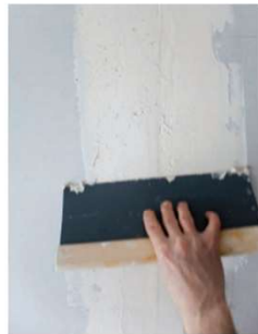
6 The filler is worked along the joint so that it finishes as flat to the surface of the plasterboard as possible.
