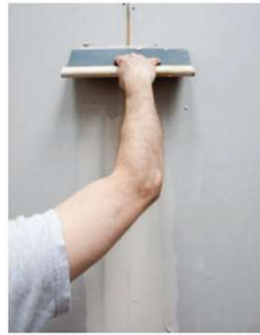
3 The first filling compound is applied to fix the tape in position.
