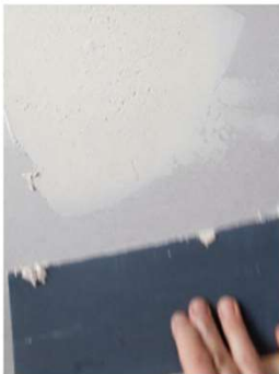
7 Heads of screws, sunken below the face of the plasterboard sheet, are covered with dabs of filler that are then roughly levelled by hand.
