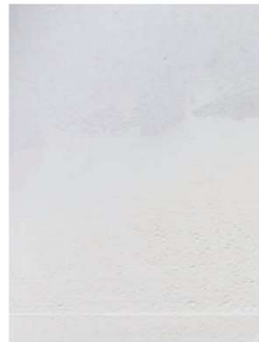
9 The filler is sanded to eliminate the slight pitting that follows the hand-leveling process, and to reduce further any filler that remains above the level of the plasterboard.
